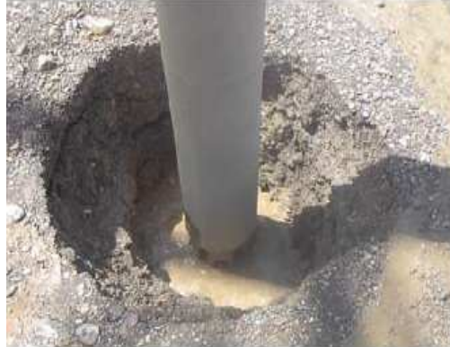
Figure I.11: Liquéfaction du sol.
